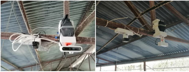
Fig. 2. Photos of the monitoring system.
